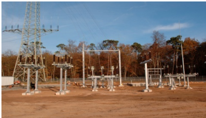
Power grid connection
