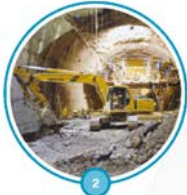
2 CIVIL ENGINEERING 2 new caverns and two new 300-metre service galleries, two new large shafts; 10 new technical buildings on surface in P1 and P5 (ATLAS and CMS)
