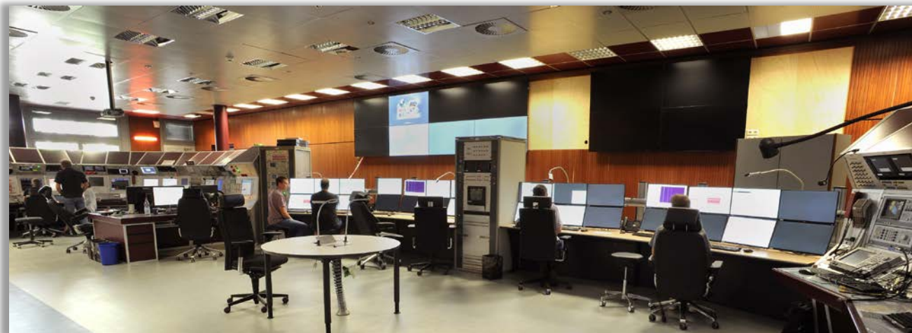
Central control room with new FAIR console environment (June 2018)
