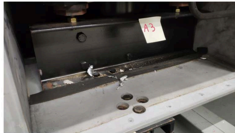
A3 transformer air box detail – contamination with metal pieces images: B. Schlitt
