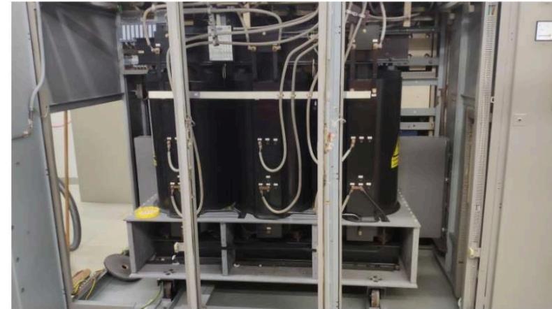
Example: A3 transformer (weight about 3.6 t)
