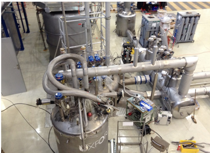
precooler and distribution box
