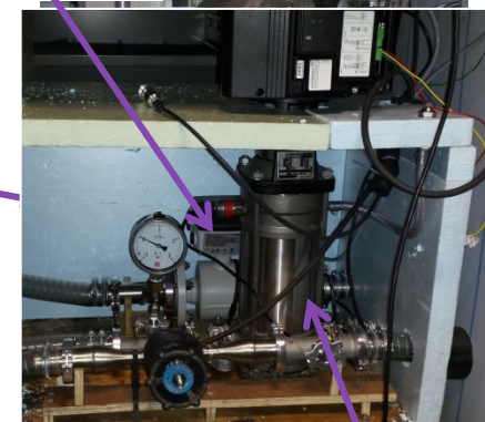
Pump circulator of the chiller
