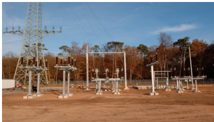
Power grid connection
