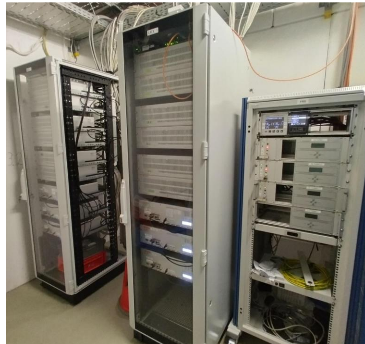
New Cosylab hardware (FAIR standard) installed in new room
