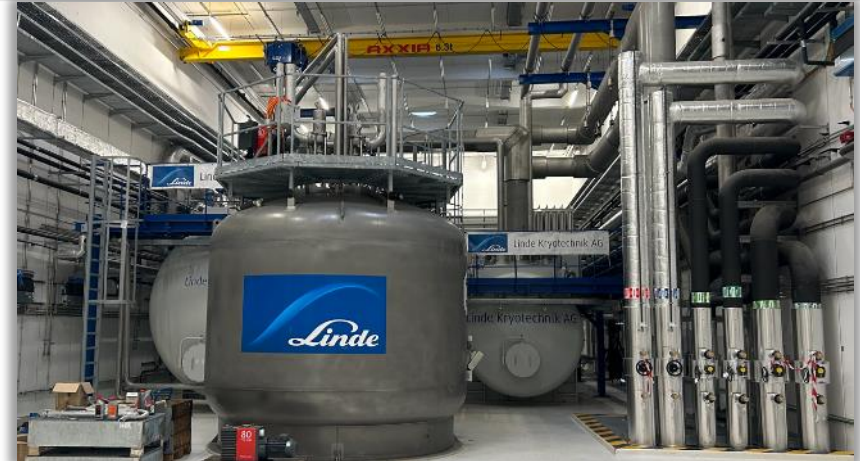
FAIR Cryogenic plant “Cryo2” and Distribution box 3
