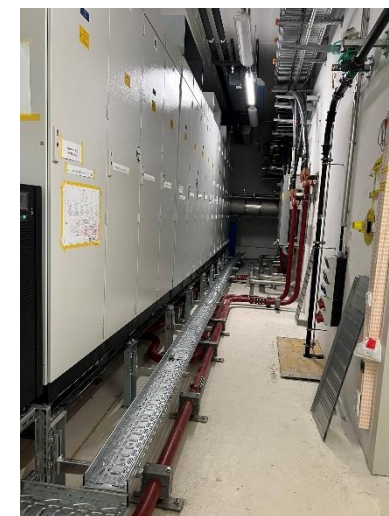
Installation of Racks for the SIS100 Main power supply at level U20
