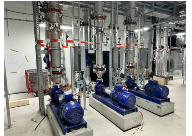
■ H0719A, cooling water distribution
