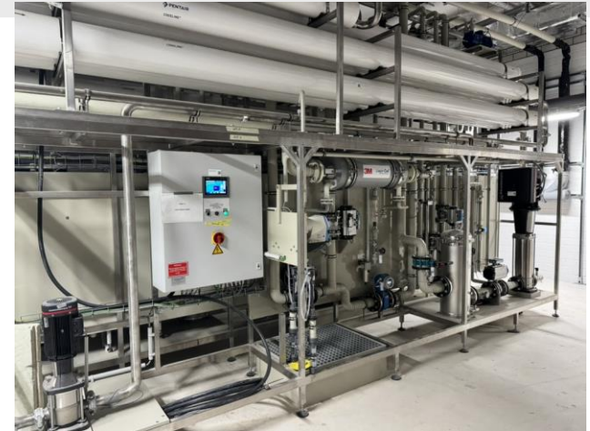
■ H0719A, water treatment
