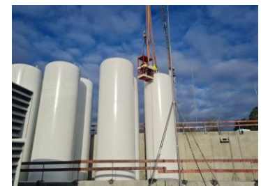
100m 3 warm gas helium storage tanks
