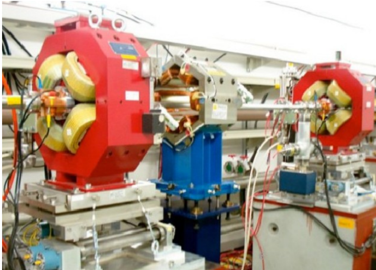
SK1 placed between QF5 and QD6
