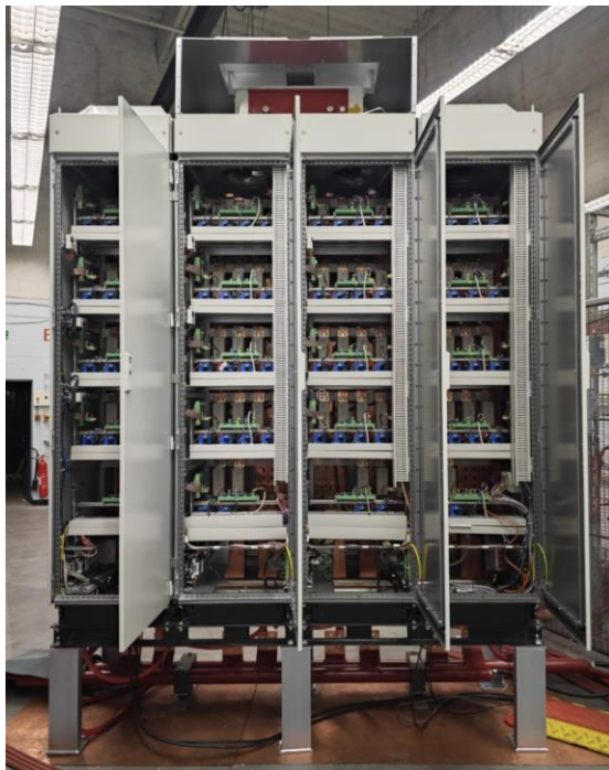
4 T/s operation – 14.5/11.5 kA
