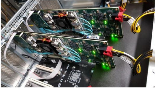
2 CRI cards installed in one entry node
