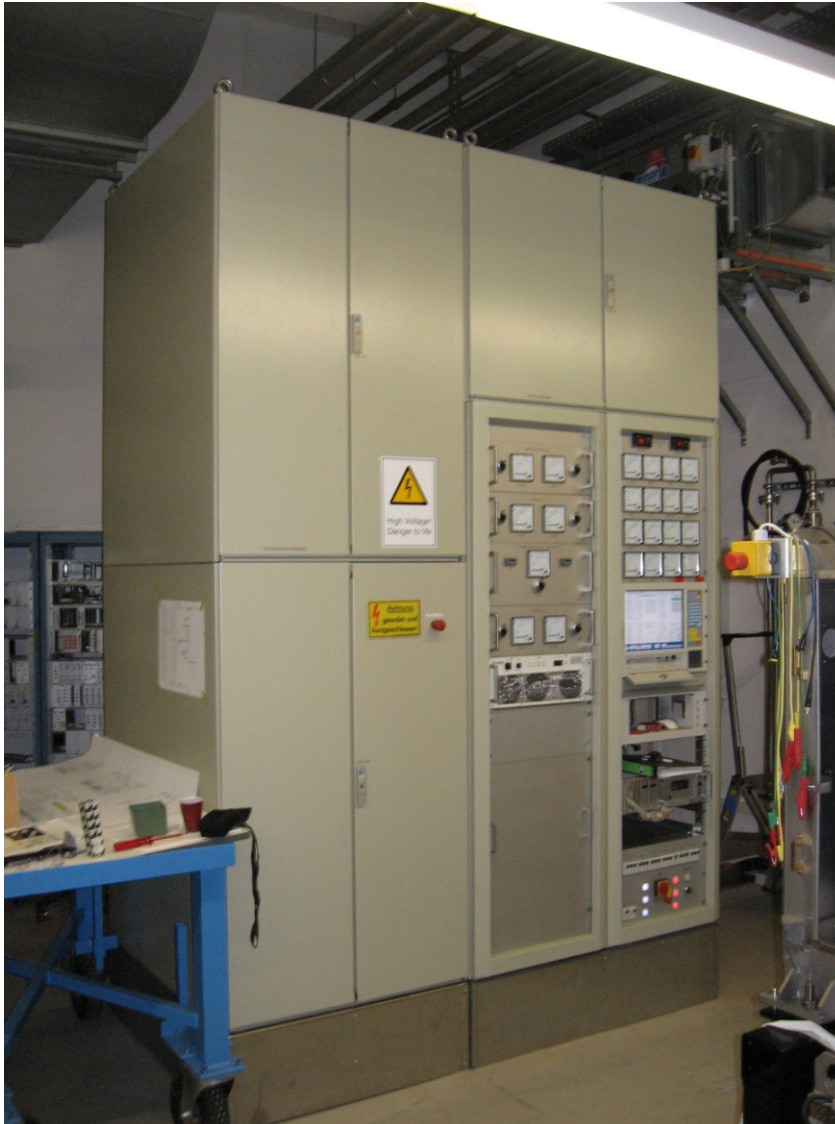
Supply Unit of SIS18 Bunch Compressor, GSI
