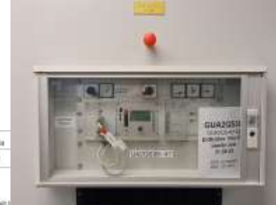
A2QS105+106 out of operation
