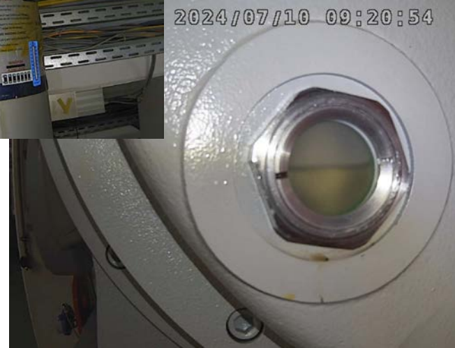
pump bearing oil reservoir
