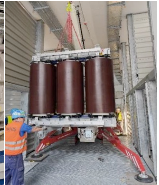
Installation of transformers and switch gears of the main power supply of the Dipole Quadrupole Magnets
