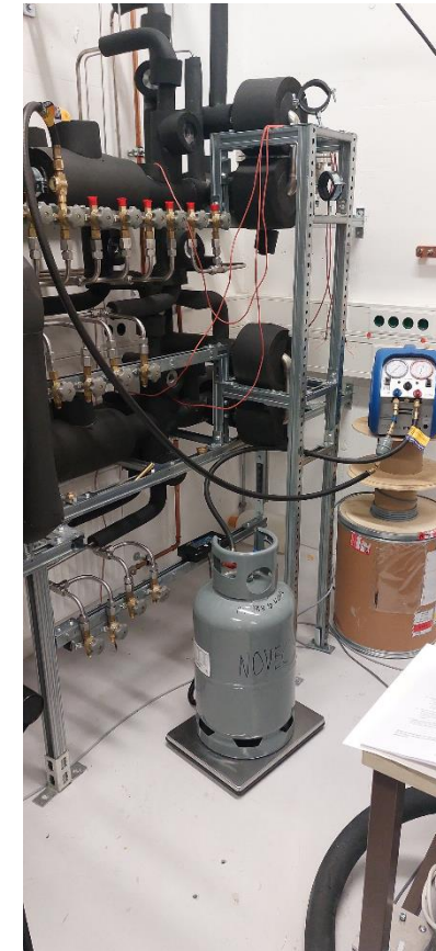
The drainage system connected to the cooling test rig
