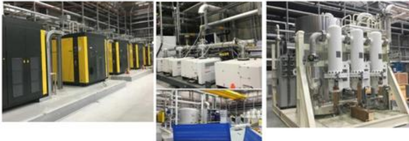
Compressors and Oil Removal System (WCS)
