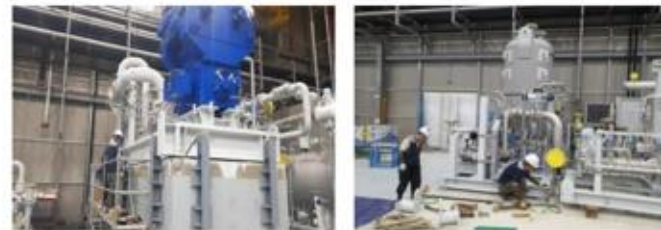
Compressors and Oil Removal System (WCS)
