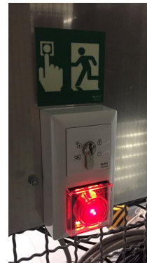
Escape Route System Terminal Area 1
