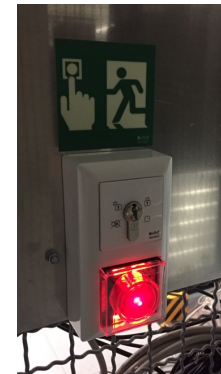
Escape Route System Terminal Area 2
