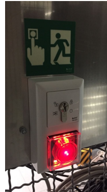
Escape Route System Terminal
