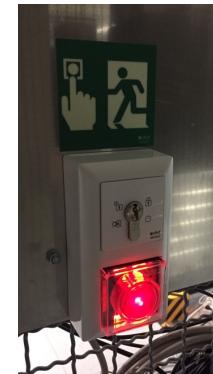
Escape Route System Terminal
