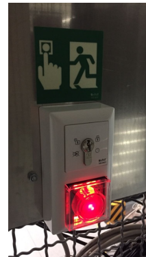
Escape Route System Terminal
