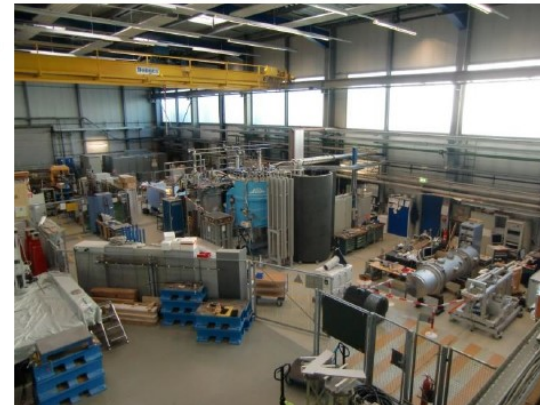
Preparation area, Cryogenic infrastructure is located in the middle of the hall
