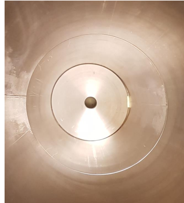
Picture 11: 2 x Vacuum pipes welded view inside Wall thickness 2 mm Inner diameter 140 mm
