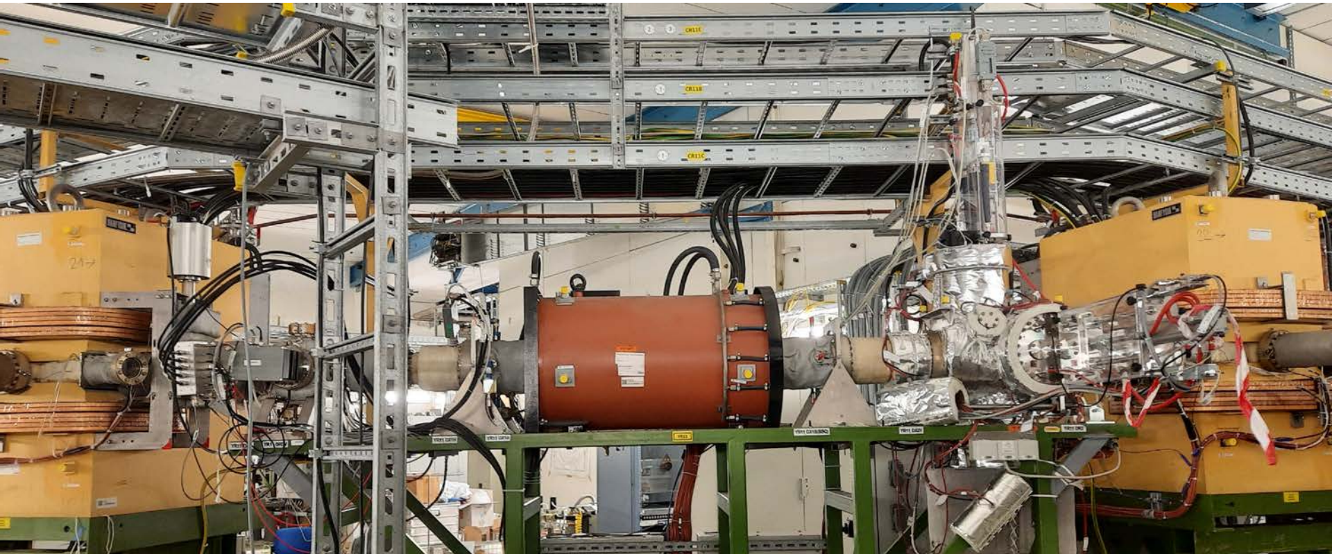
Dipole vacuum chambers with straight port
