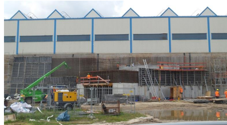
Interface for FAIR tunnel 101
