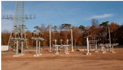
Power grid connection
