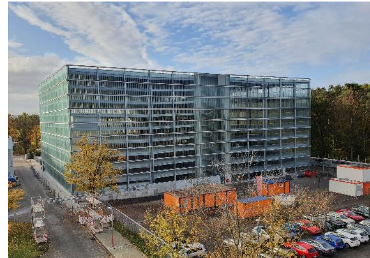
Picture showing the current status of civil works of the parking garage 3 rd November 2020.
