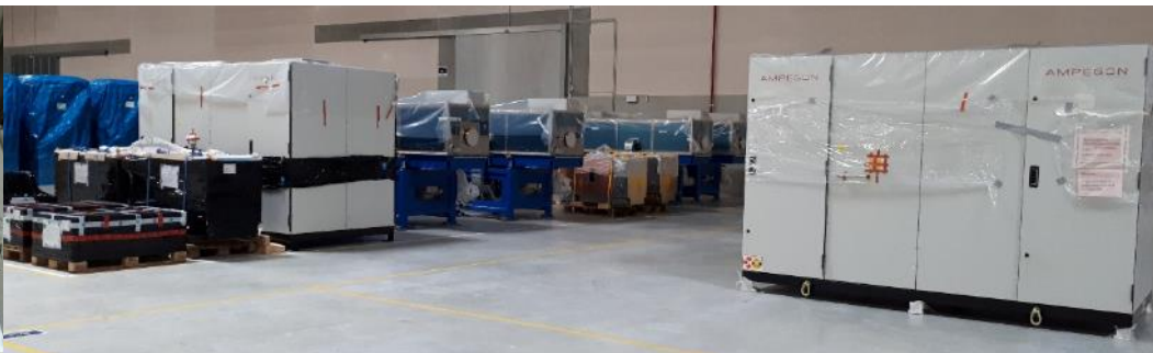
Rf acceleration cavities and power converter in storage are
