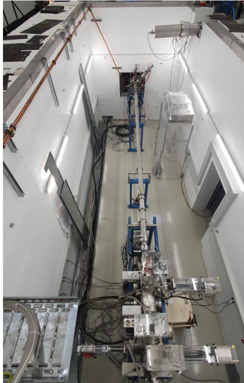
New Testbunker with test bench (2020)
