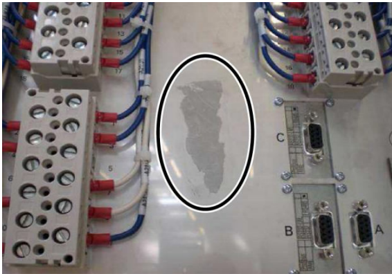
Fig. 87: Unwanted adhesive residues
