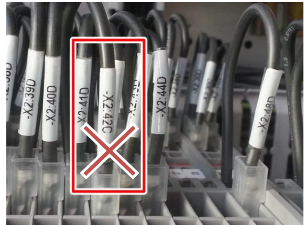
Fig. 43: Wire identifications must all be affixed with the same text alignment.
