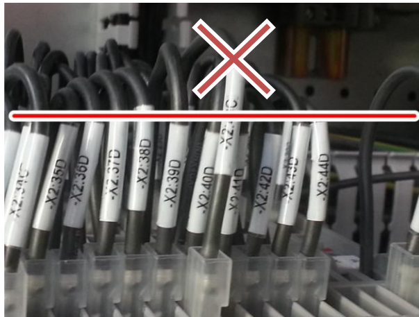
Fig. 42: Wire identifications must all be affixed at the same height with an even distance from the clamps.
