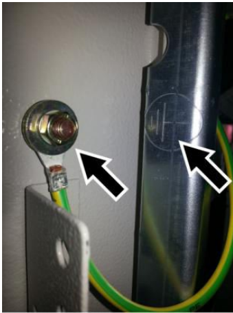
Fig. 14: Grounding cable between door and cabinet wall
