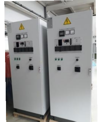
Sextupole & steerer power converters
