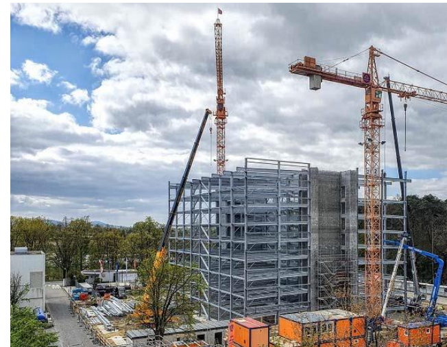
Picture showing the current status of civil works of the parking garage mid-April 2020.
