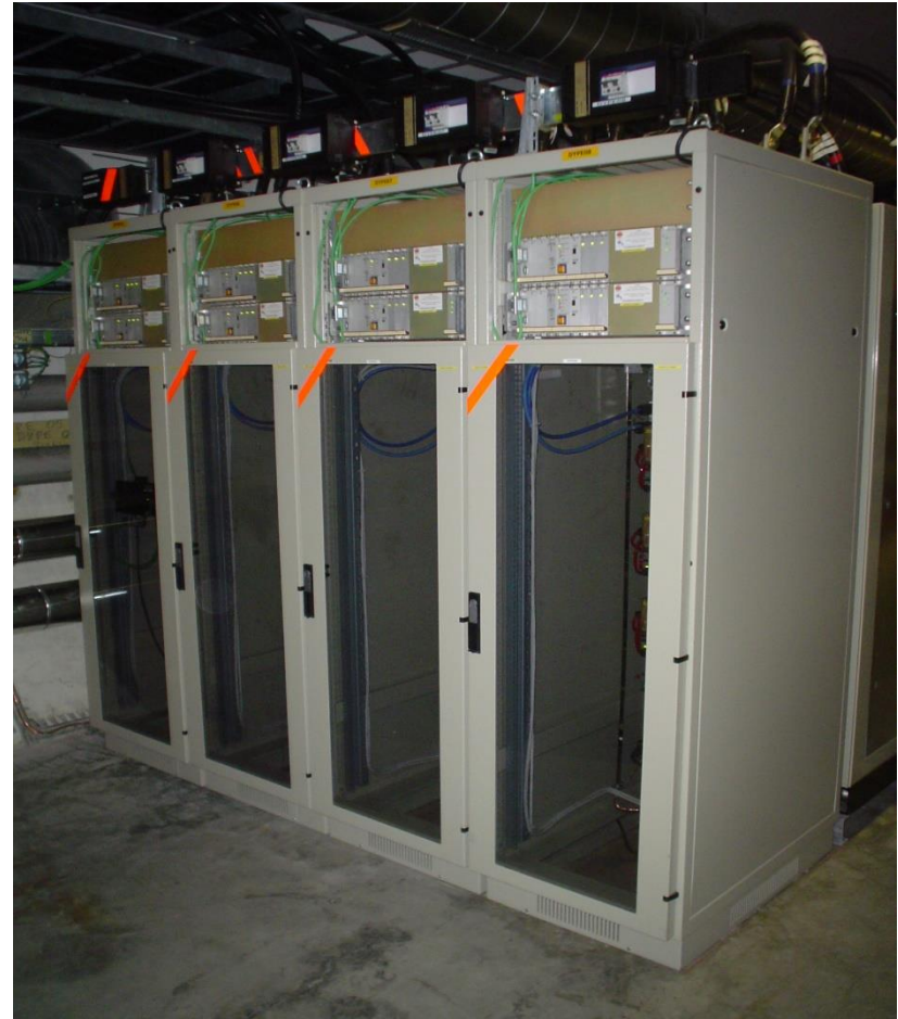
Racks in the LHC tunnel
