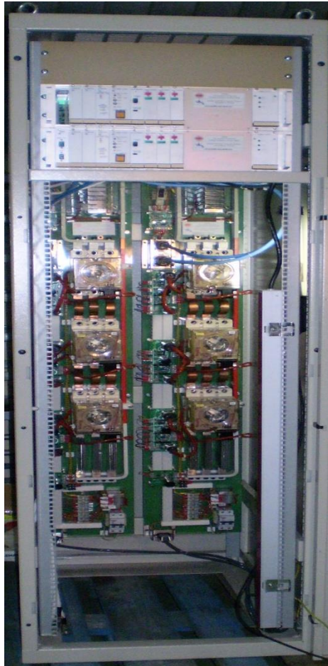
Two systems per rack
