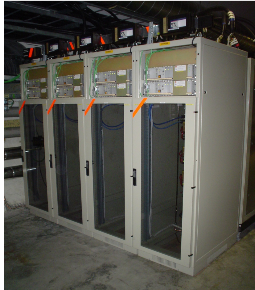
Racks in the LHC tunnel
