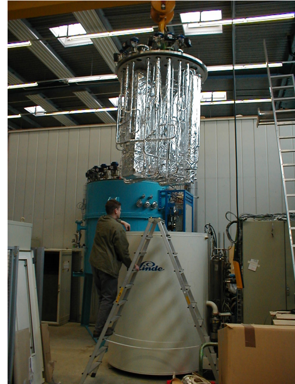
picture of the interior of a very similar cold-box of a cryogenic plant
